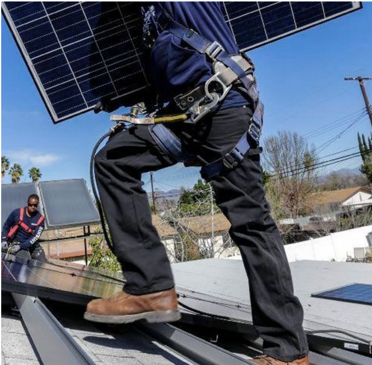
Alejandro DeLeon carries a solar panel as crew members from Sunrun home solar company install a solar system on a home in Van Nuys in 2016. (Irfan Khan / Los Angeles Times)
