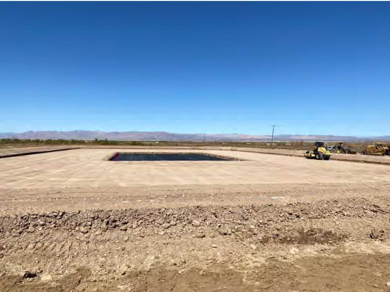
Well pad construction at the site of Controlled Thermal's planned geothermal and lithium facility. (Rod Colwell)
